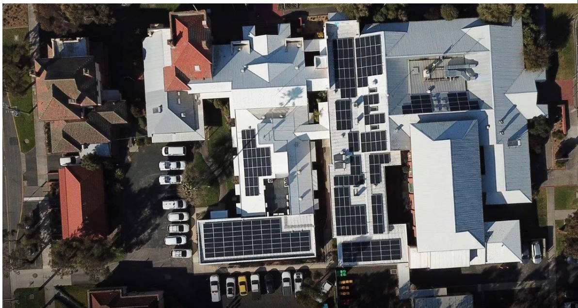
100kW PV rooftop solar system installed on the Wonthaggi Civic Centre.
