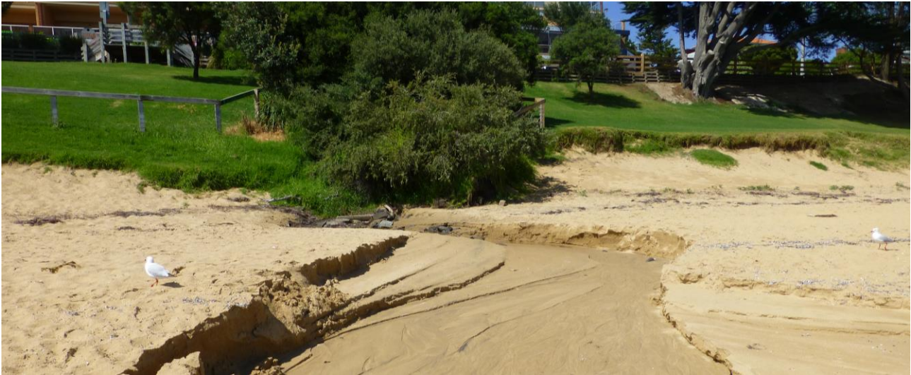
Figure 2-5 Storm water outfall located on Cowes main beach.
