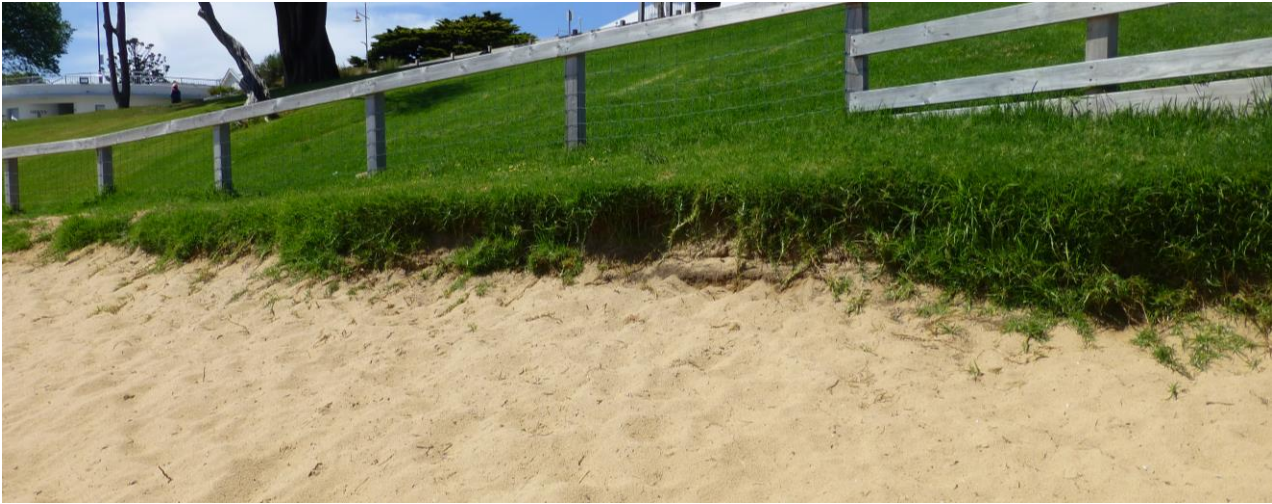
Figure 2-2 Erosion scarp at beach interface with foreshore reserve
