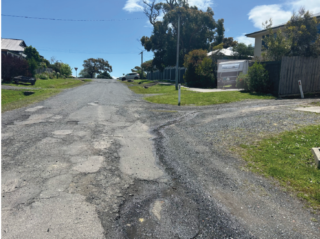
Image 2: Deterioration along Queen Street, between Merrin Crescent and Broome Crescent.
